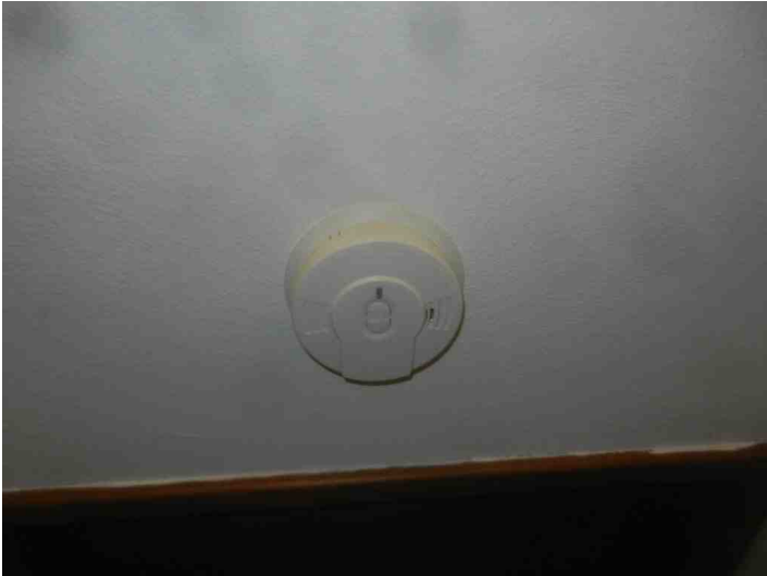
Smoke & CO detector
