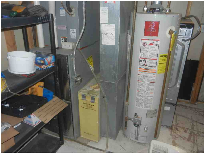
Furnace & water heater
