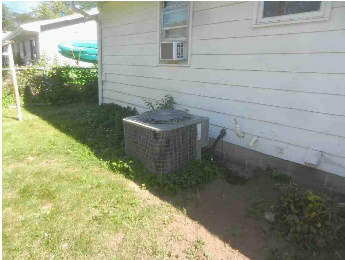
Central air unit
